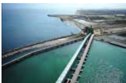
View from the pier: the last section of the Pipe Conveyor runs along the sea to the transfer tower.
