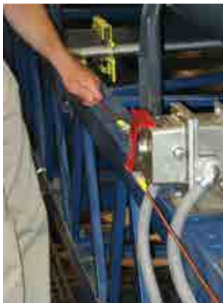
SAFETY EQUIPMENT SUCH AS PULL STOPS AND EMERGENCY SWITCHES ARE VITAL TO CONVEYOR SAFETY © MARTIN ENGINEERING 2021
