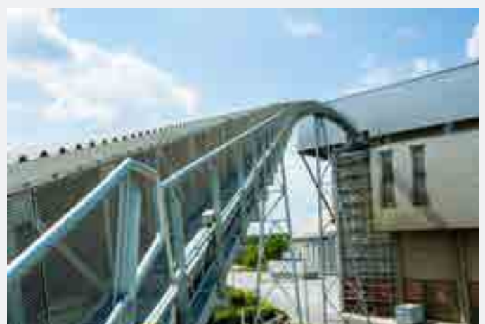
A PIPE CONVEYOR: THE ENCLOSED SYSTEM ENSURES ENVIRONMENTALLY SAFE, DUST-FREE AND LOW-ENERGY TRANSPORT OF THE ALTERNATIVE FUELS (© BEUMER GROUP GMBH & CO. KG)
