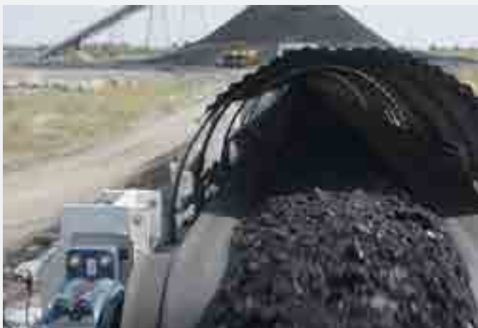
THE OVERLAND CONVEYOR TRANSPORTS THE COAL FROM THE MINE TO THE MAIN PROCESSING PLANT (© BEUMER GROUP GMBH & CO. KG)
